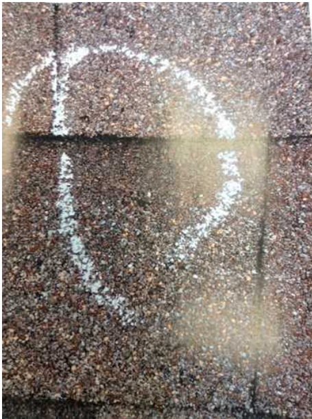
Close-up - Roof - Front - Damaged - Hail
