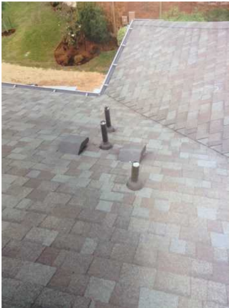
Vents - Overview - Roof - Right - Damaged
