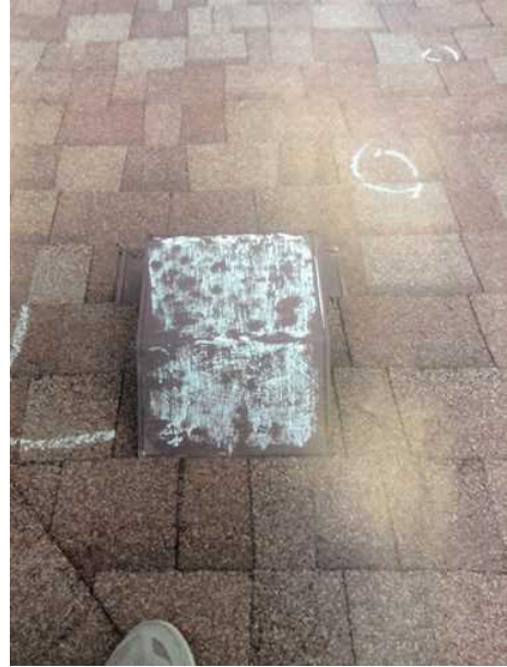
Close-up - Roof - Back - Damaged - Hail
