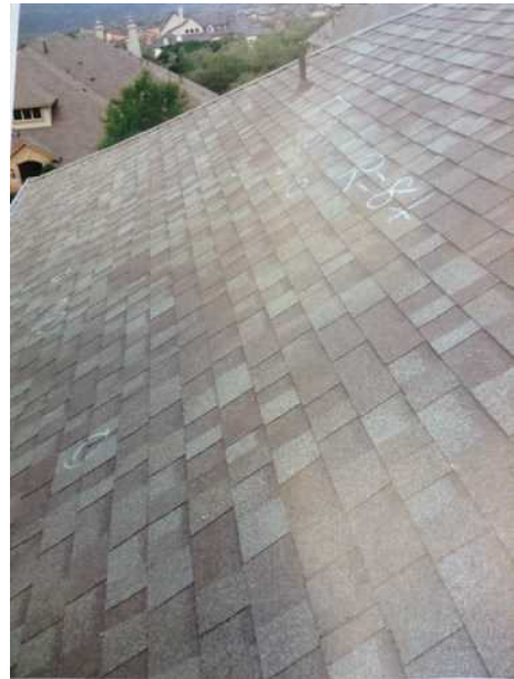
Overview - Roof - Right - Damaged - Hail - Hail Hits: 8
