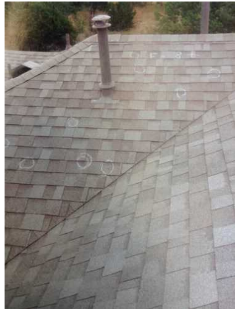
Overview - Roof - Front - Damaged - Hail - Hail Hits: 8
