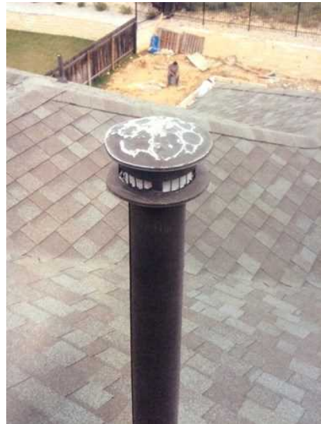
Exhaust Cap - Close-up - Roof - Back - Damaged - Painted
