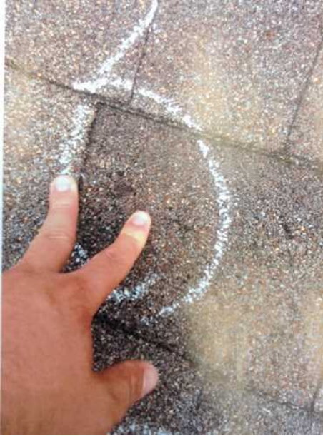
Close-up - Roof - Right - Damaged - Hail
